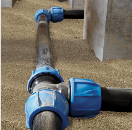
Water Distribution Lines
